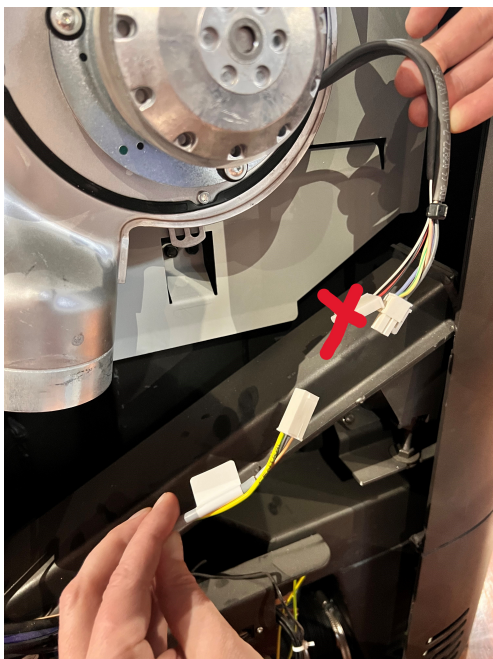
Fig. 23: Connecting the cables
